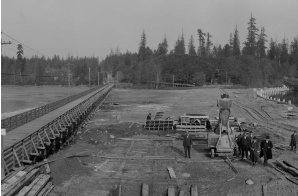
Fig 14. Crews working on the construction of the causeway. Detail from “Coal Harbor Vancouver. Height of Water in Upper End 9 ft. above. Zero,” November 6, 1917. Major Matthews collection, AM54-S4-3-: PAN N54, City of Vancouver Archives.
